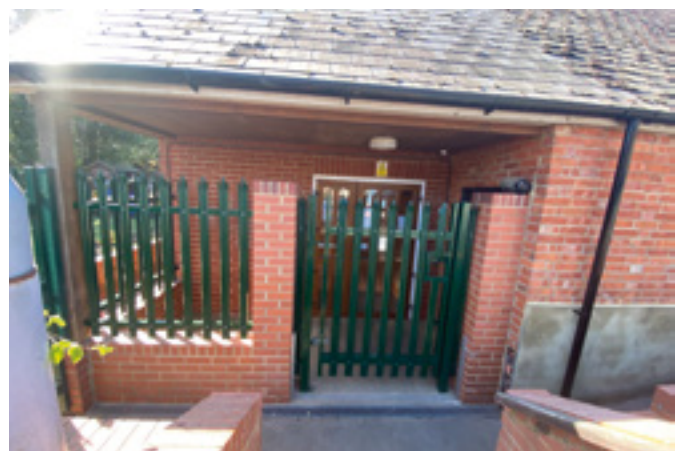
Security fencing at Crowthorne Parish Hall to prevent anti-social behaviour and vandalism
